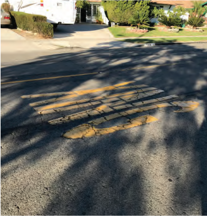
Fading school pavement markings on Woodbury Ave.
