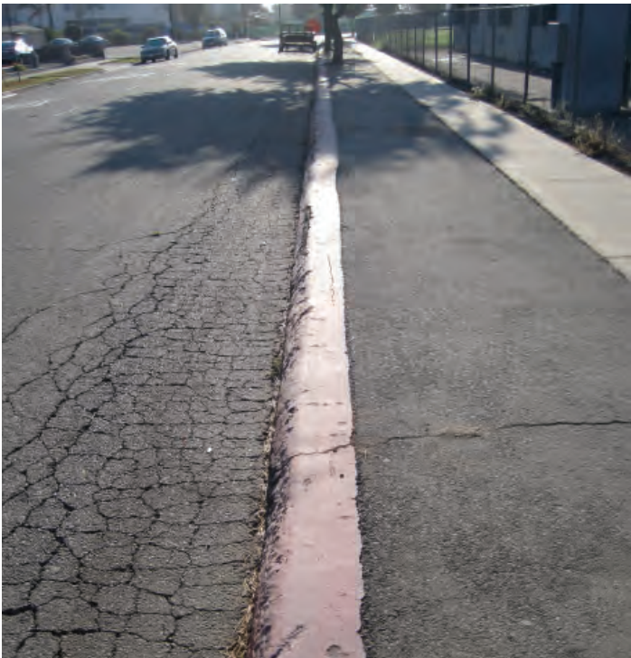
Cracked pavement on Bixby Avenue with wide sidewalks adjacent to the back entrance of the school.
