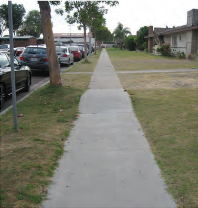
Uneven sidewalk along Washington Avenue.
