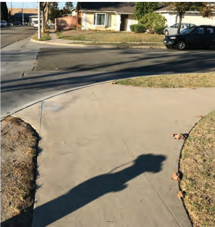
Lack of ADA-compliant curb ramps on Woodbury Ave.
