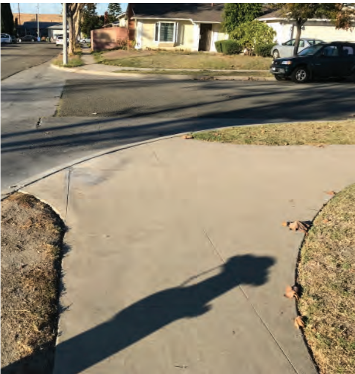
Missing ADA-compliant curb ramps along Erin Street.
