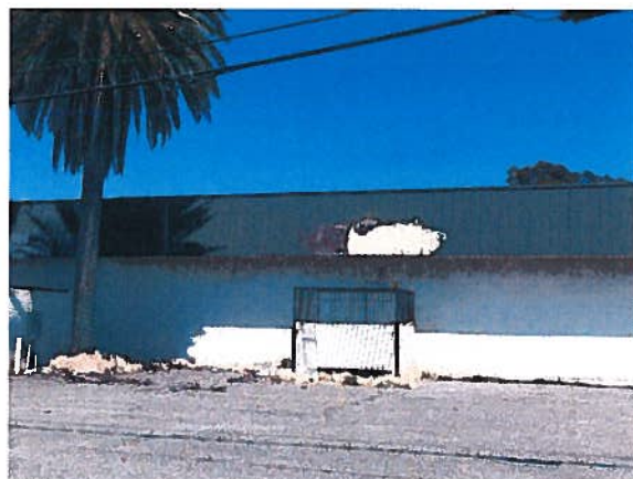
Damage and unusable trash enclosure along with overgrown vegetation
